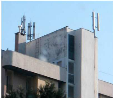
FIG: Antenna system of GSM base station mounted on a roof top at the altitude of approximately 17m above ground.
